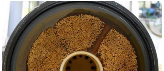
Typical Iron fouling
