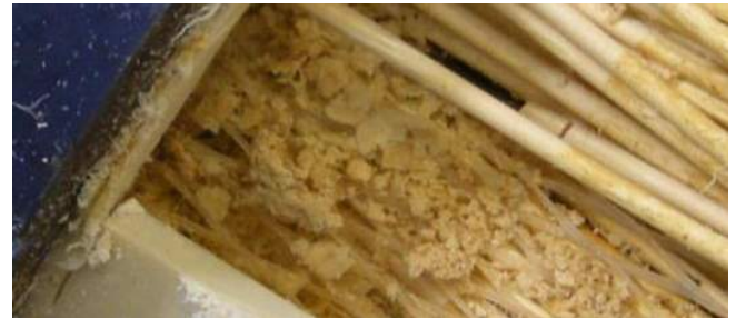
Carbonate scale deposits
